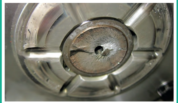
Fatigue crack - pump side
